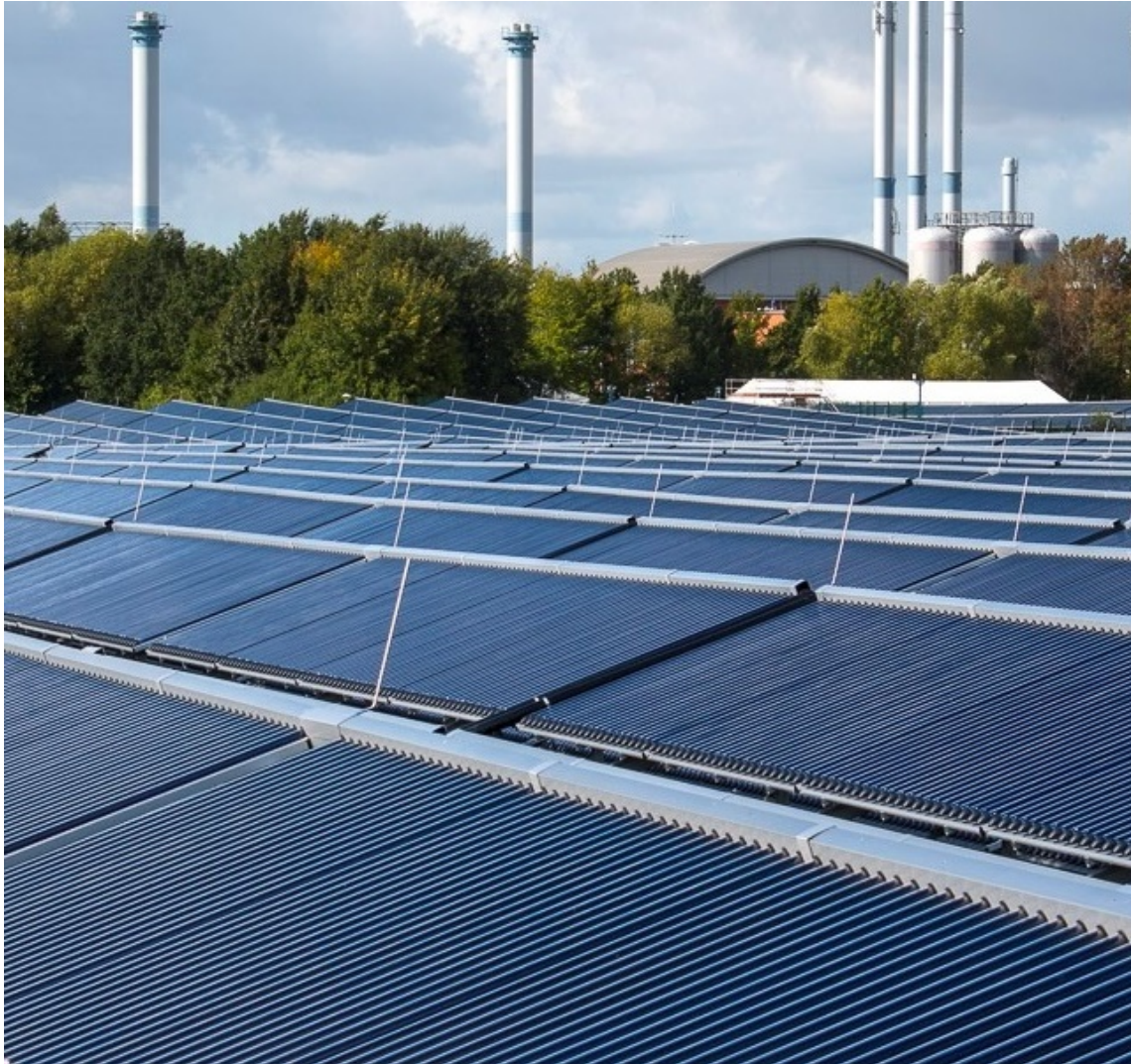
iKWK-System Greifswald (18.732 m 2 ) (Foto: Guido Bröer)
